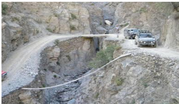
Fig. (4). Unstable roads in the mountainous region of Chitral
